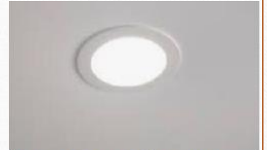
RECESSED LED LIGHTING OVER DINING TABLE
